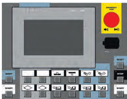
CONTROL PANEL: SIEMENS (X)
